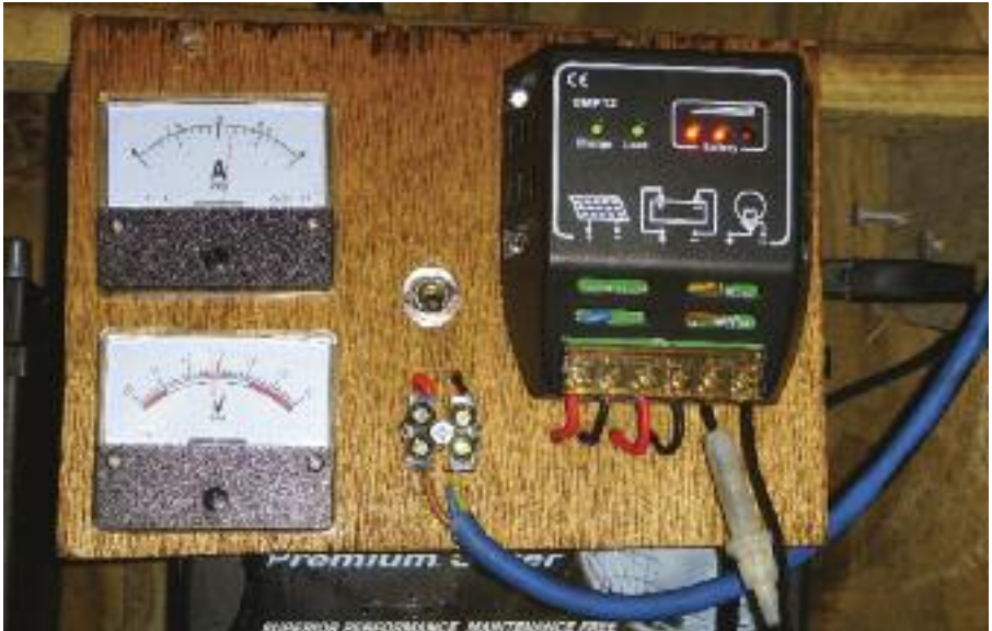
Figure 3 the Control Board with battery behind Photo: Charlie Cartwright
